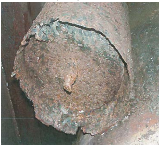
Corroded Spring Hanger
